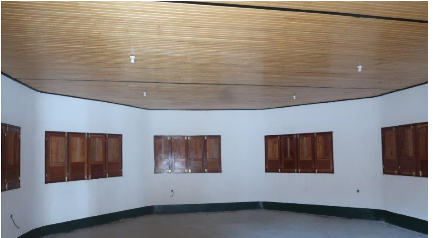
Office of Ndima Kali and library inside the PAPA building © Luis Arranz
