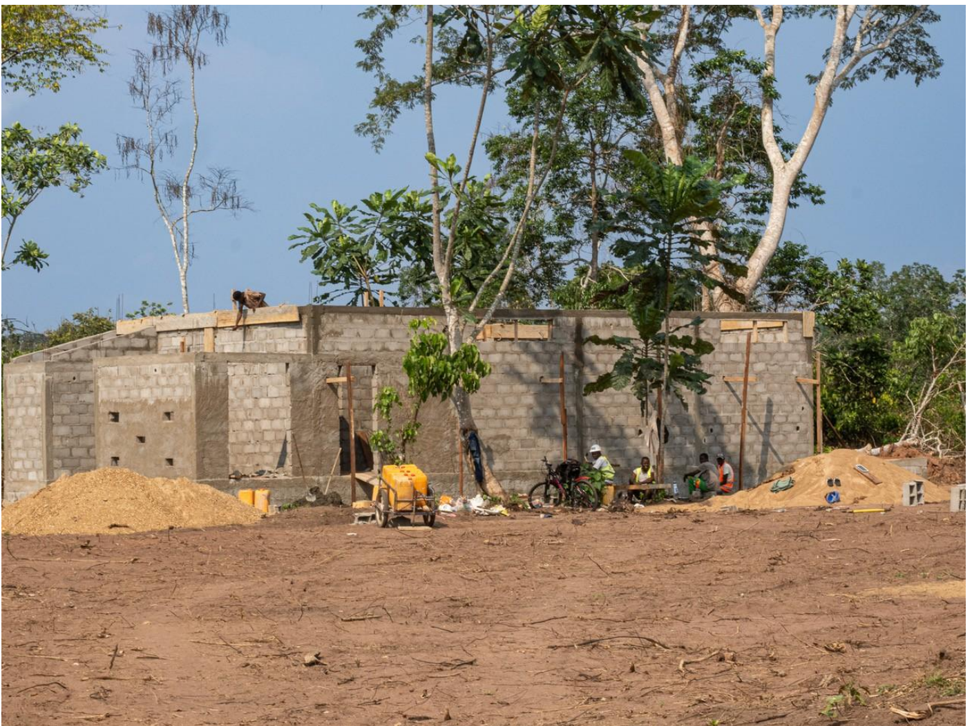
The works of the new solar central has finally started © Nuria Ortega
