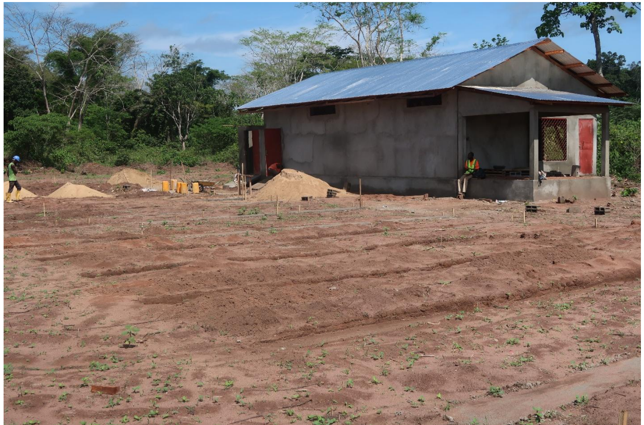
The construction of the central of the solar system advance, slowly, but it does © Luis Arranz
